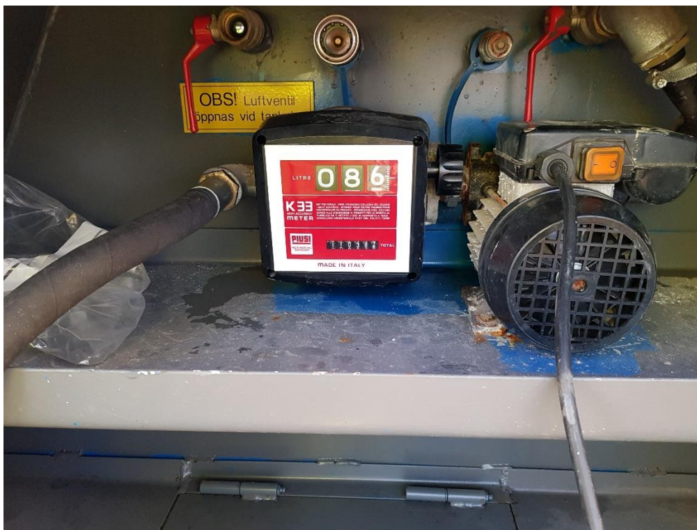
Figure 7. Reading on fuel meter after day 1, week 1. Standard mode with high frequency; 86,5 liters.
