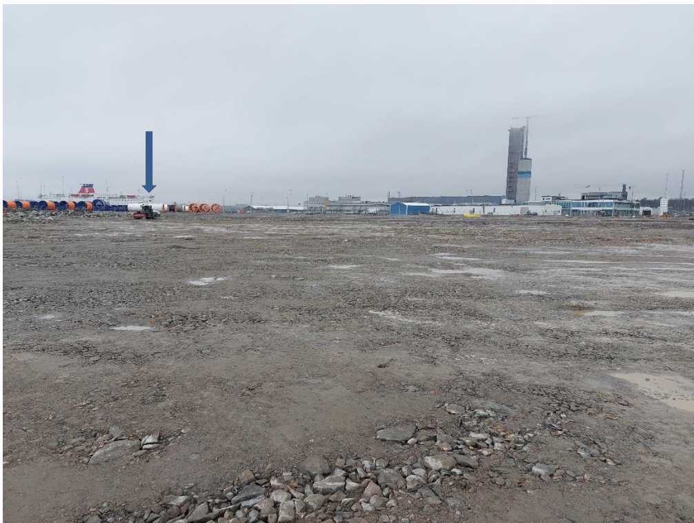
Figure 19. A view over the working site. The roller is to the left just below the horizon (below the arrow).
